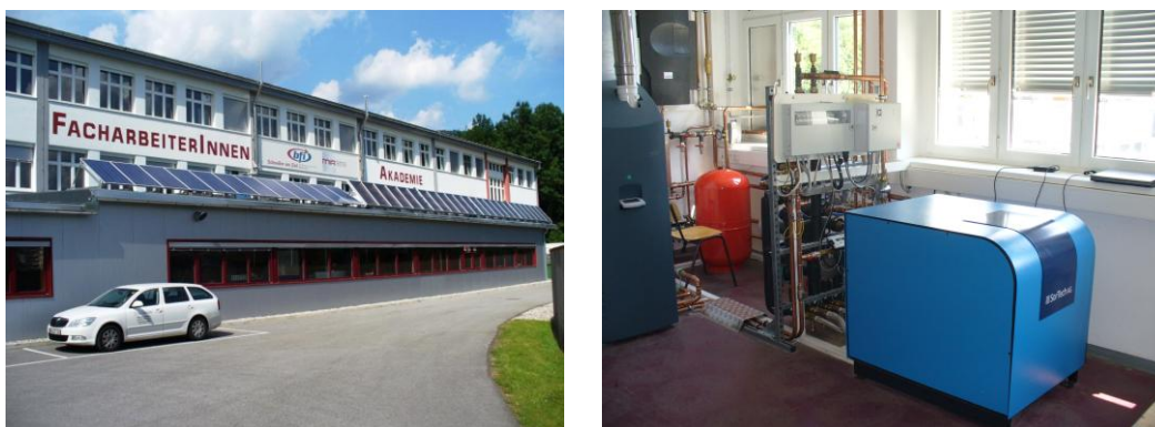
Figure 3: Solar Cooling Professional School, Mürzzuschlag, Austria (left: Solar thermal collector; right: Adsorption Chiller ACS08)
